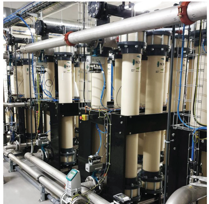
dNF installation that produces drinking and process water in one step from highly colored surface water.
